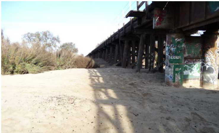
Figure 2-9. Sediment Accumulation within Paradise Cut Reducing Bypass Capacity (Photo taken December 3, 2012)
