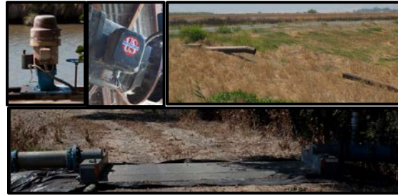
Figure 11. Images of diversion and return locations, clockwise from the top left corner: active diversion pump; inactive diversion pump depicting cut wires; inactive siphon depicting pipe separations; and temporary diversion, depicting flat piping laid over a levee road.
